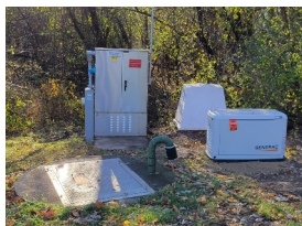
Lift Station 4 Generator
