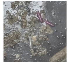
Tampon applicators floating in Lift Station 6.
