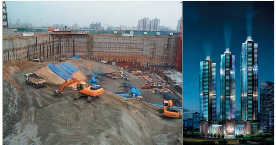
Fig. 7. A value engineering workshop was held when groundworks on this major, multi-storey project were significantly underway (courtesy Hyundai Engineering and Construction Company Ltd, South Korea)
