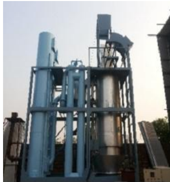
1 MW Gasification Unit
